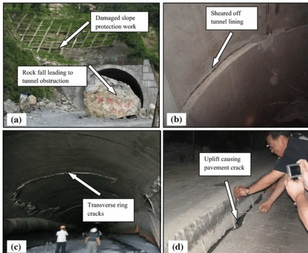
FIGURE 1. Damages at the Longxi tunnel during the 2008 Wenchuan Earthquake Source: Yu et al. (2016)
